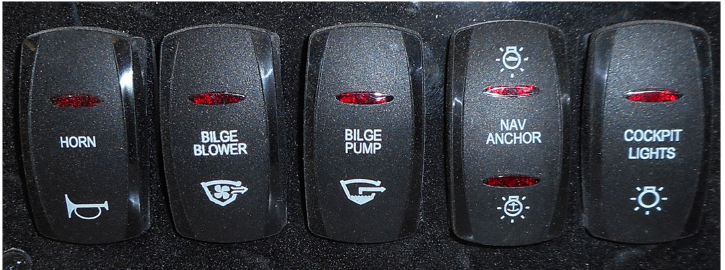
PORT SWITCH PANEL
