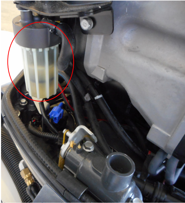
CHECKING ENGINE MOUNTED FUEL FILTER
