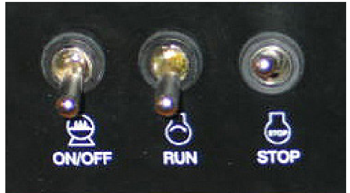
TYPICAL GEN-SET SWITCH CLUSTER- MAIN PANEL
