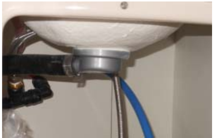
Head Sink Plumbing
