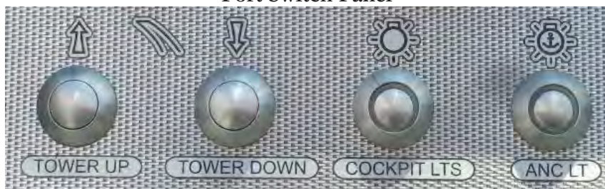
Port Switch Panel
