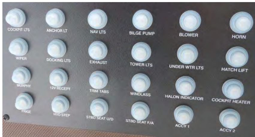
UNDER HELM BREAKER PANEL
