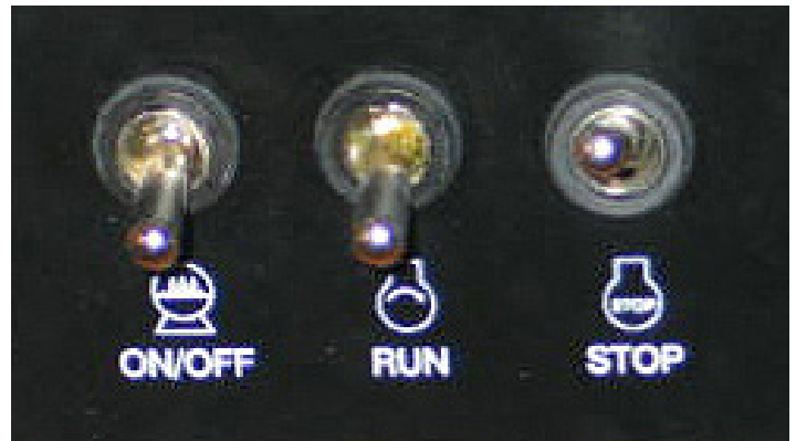
TYPICAL GEN-SET SWITCH CLUSTER- MAIN PANEL
