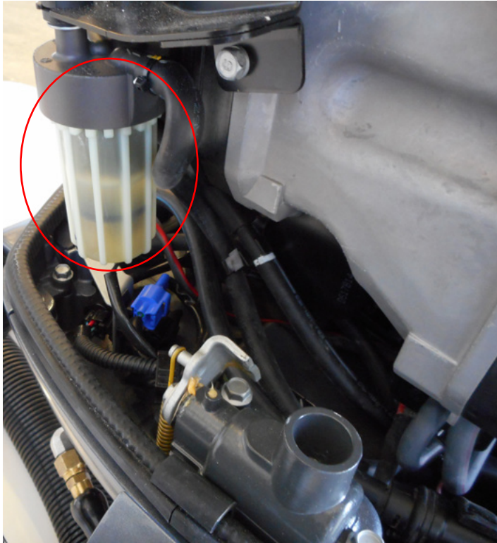
CHECKING ENGINE MOUNTED FUEL FILTER
