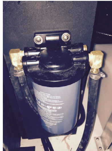
CHECKING IN-LINE WATER SEPARATOR FILTER
