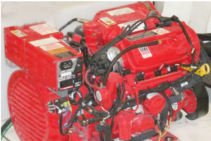
TYPICAL GAS GENERATOR
