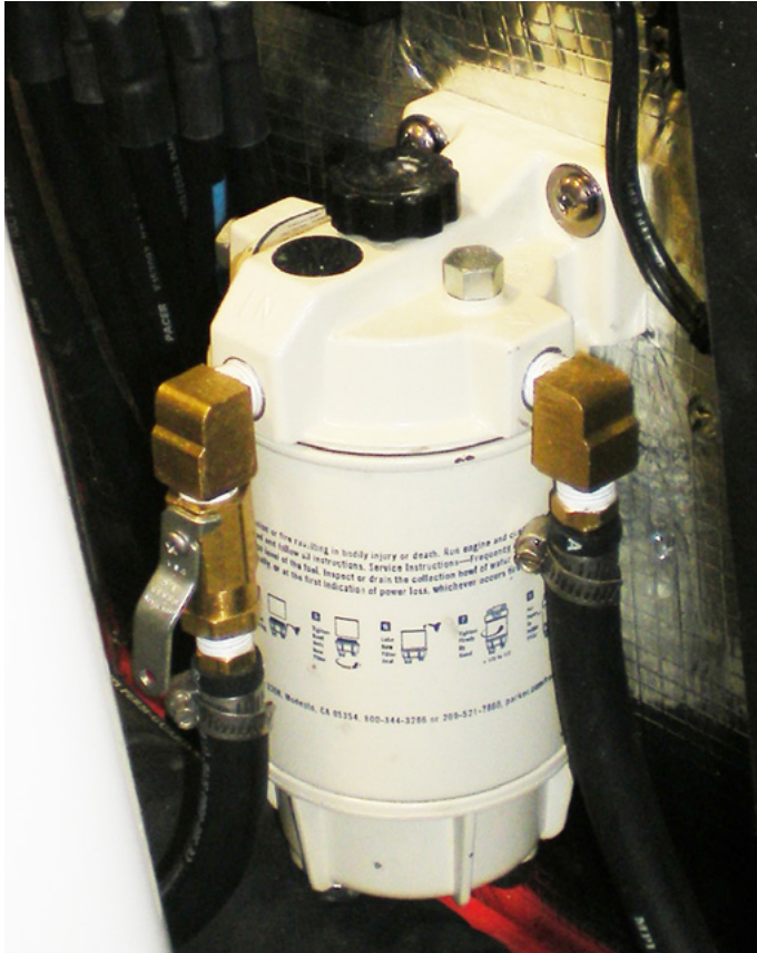
DIESEL GEN-SET PRIMARY IN-LINE WATER SEPARATOR FILTER
