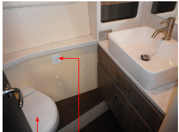
VACUUM STYLE TOILET
