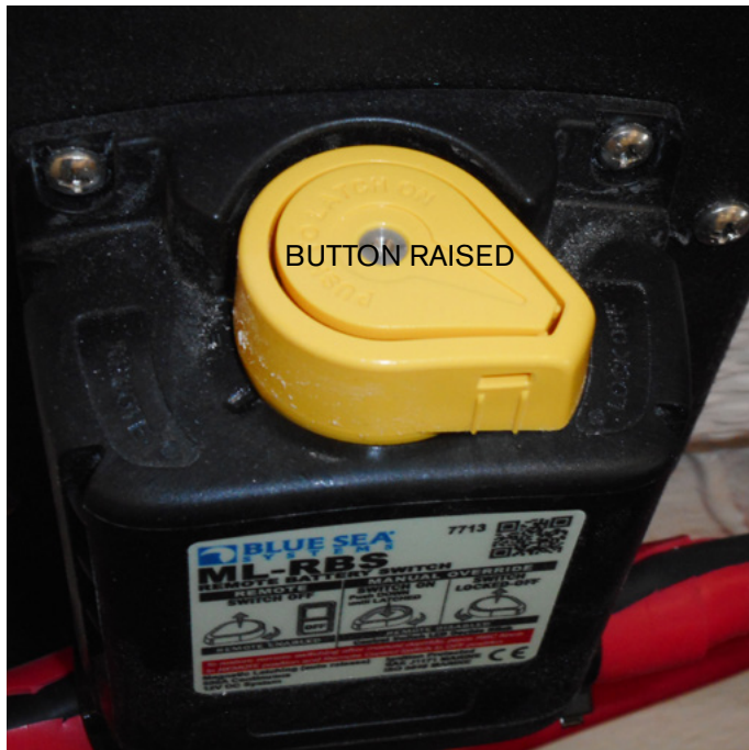
REMOTE BATTERY SWITCH- OFF POSITION
