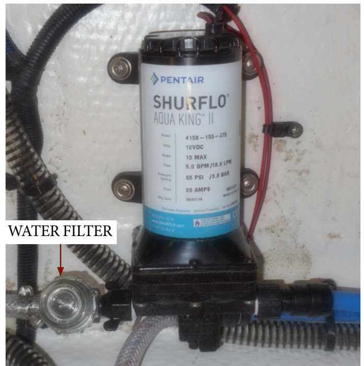
TYPICAL FRESH WATER PUMP
