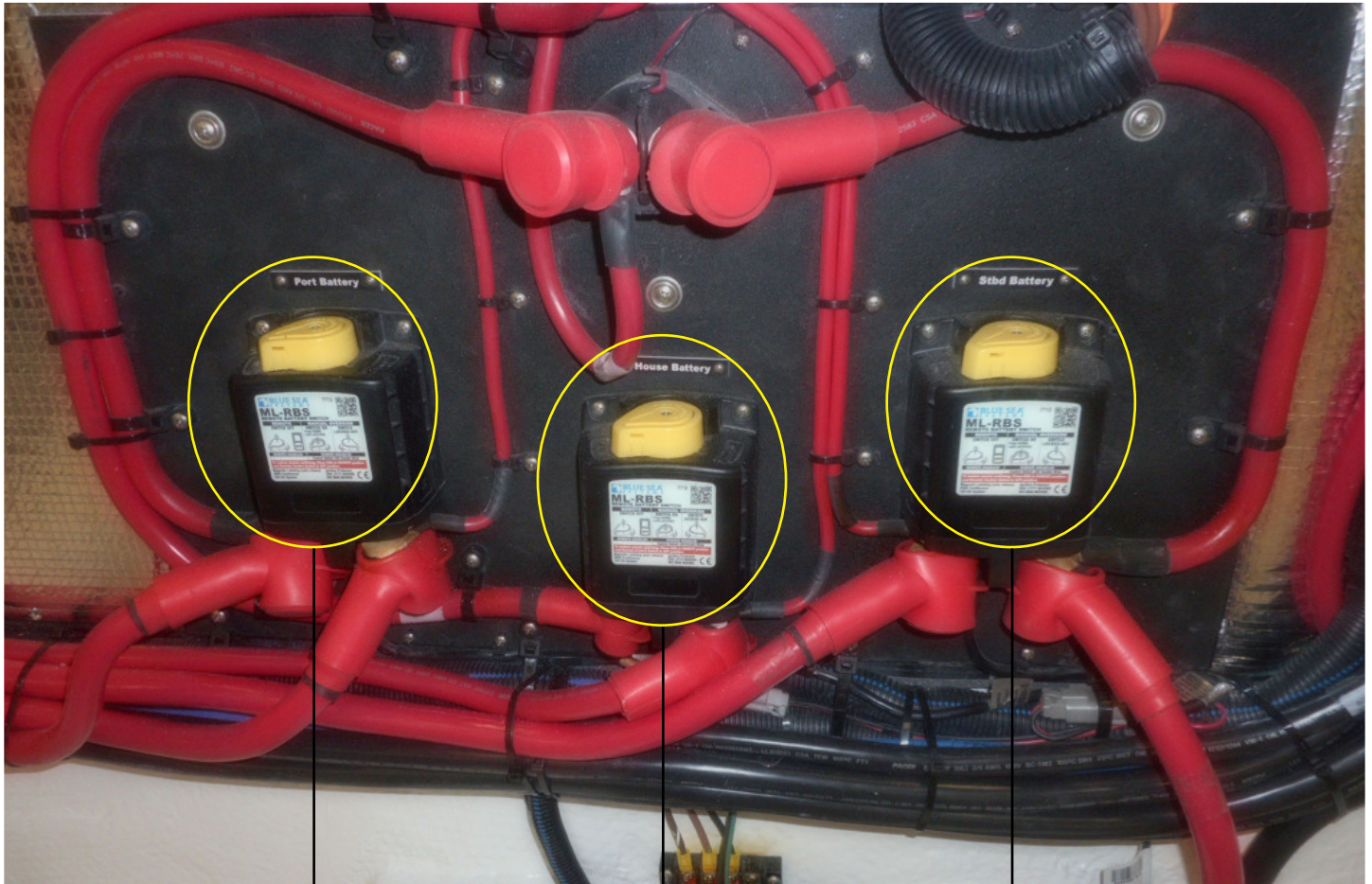
PORT REMOTE BATTERY SWITCH
