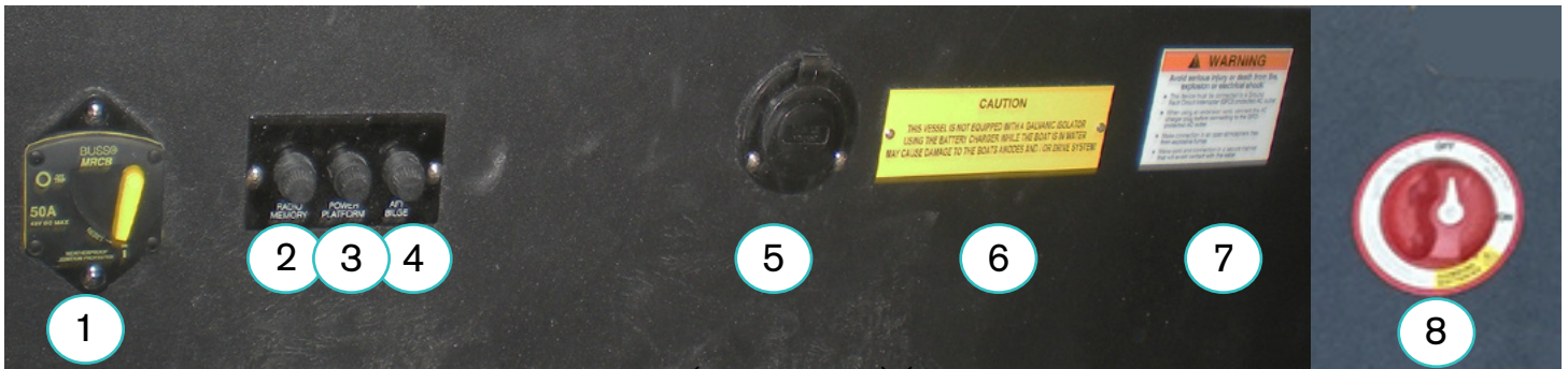
TYPICAL BATTERY MANAGEMENT PANEL (outside view) (OPT. DUAL BATTERY SWITCH SHOWN)
