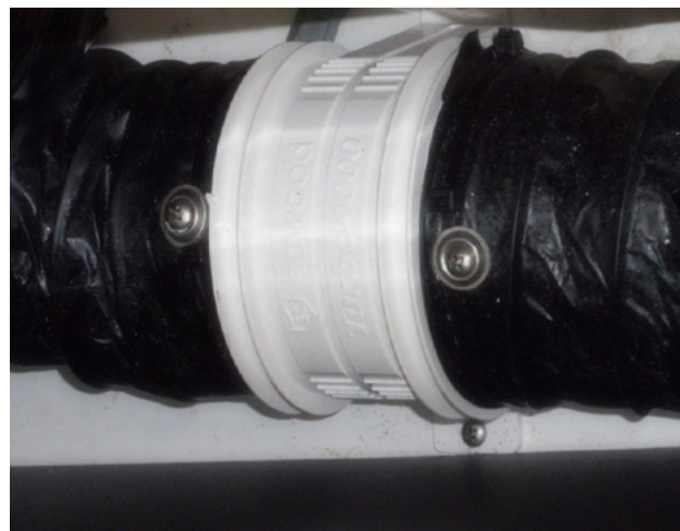
Typical Ventilation Blower with Hose
