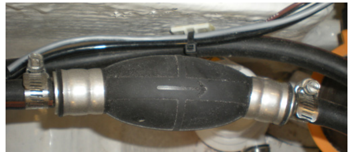
FUEL PRIMER BULB IN SUMP AREA
