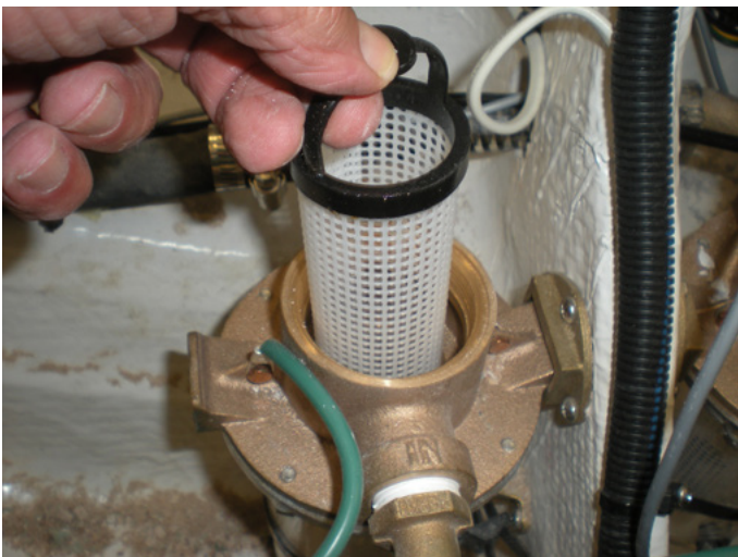
REMOVING/CLEANING STRAINER BASKET
