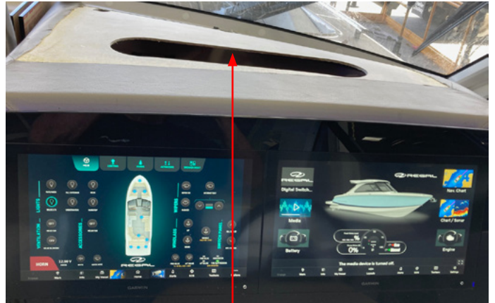
NMEA 2000 SYSTEM UNDER HELM ACCESS
