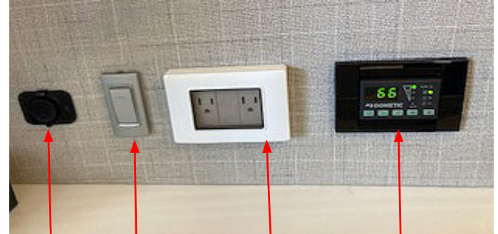
USB PORT LT. SWITCH 2 GANG ELECTRICAL BOX AC CABIN THERMOSTAT
