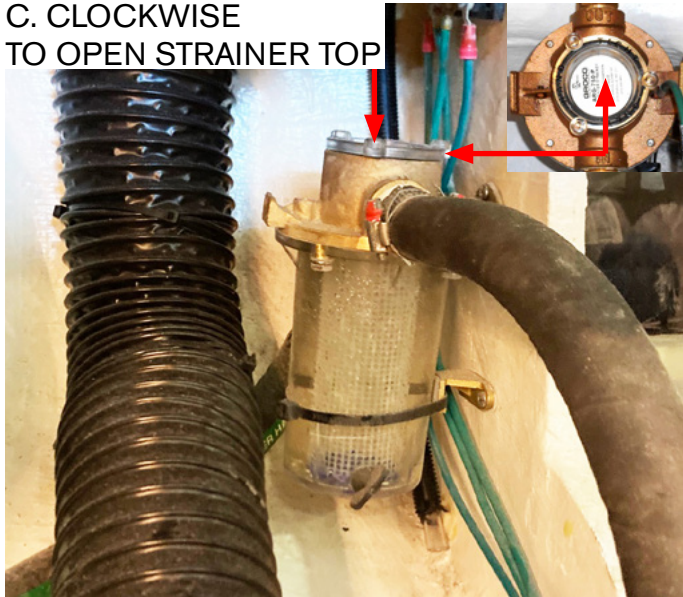
GENERATOR STRAINER W/ MESH BASKET
